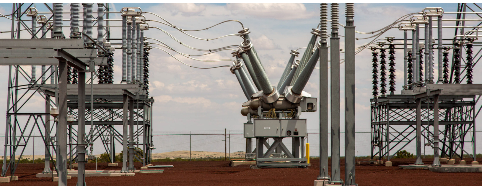
Photo Courtesy of U.S. Department of Energy – Western Area Power Administration
