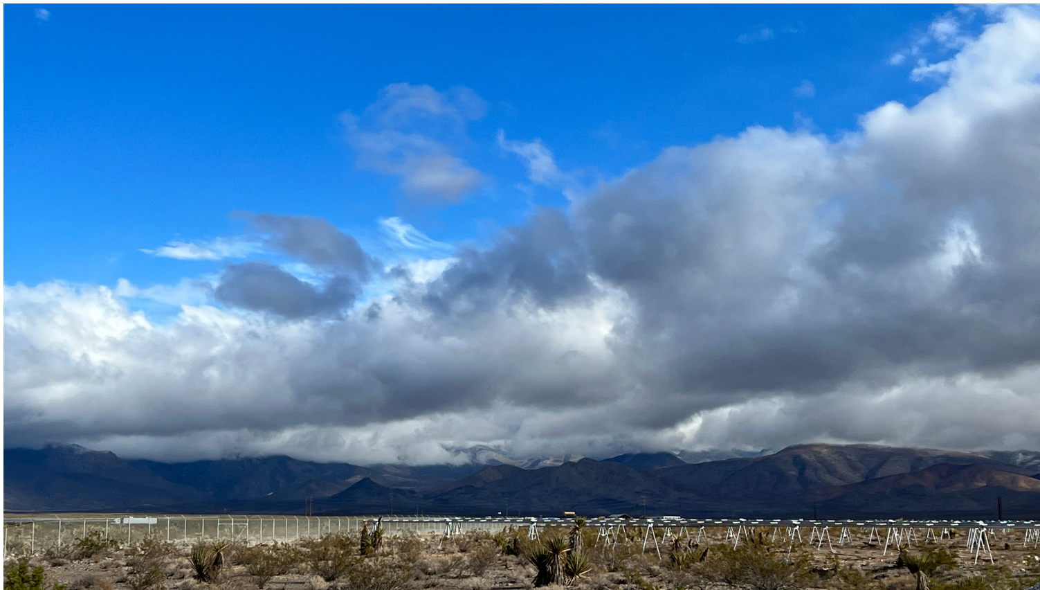
Solar panel construction outside of Las Vegas, NV Credit: Permitting Council Staff
