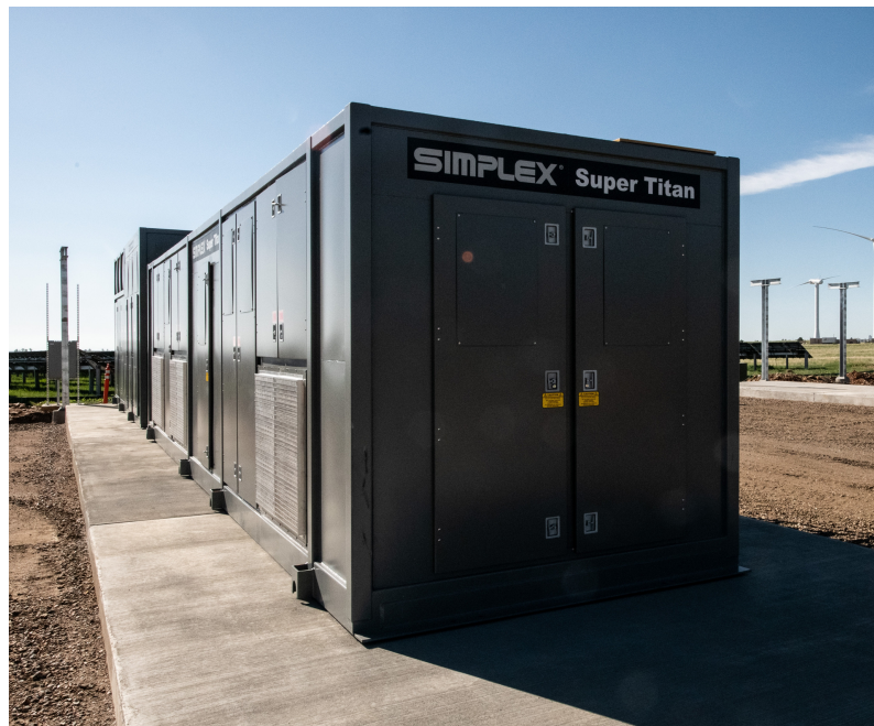
Energy storage facility. Credit: Dennis Schroeder, National Renewable Energy Laboratory
