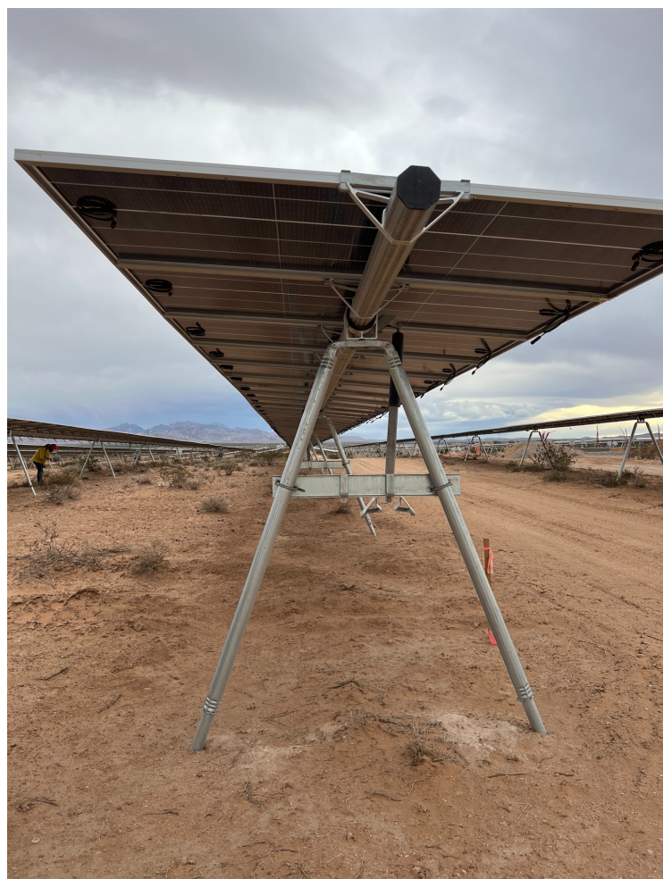
Solar panel construction outside of Las Vegas, NV Credit: Permitting Council Staff
