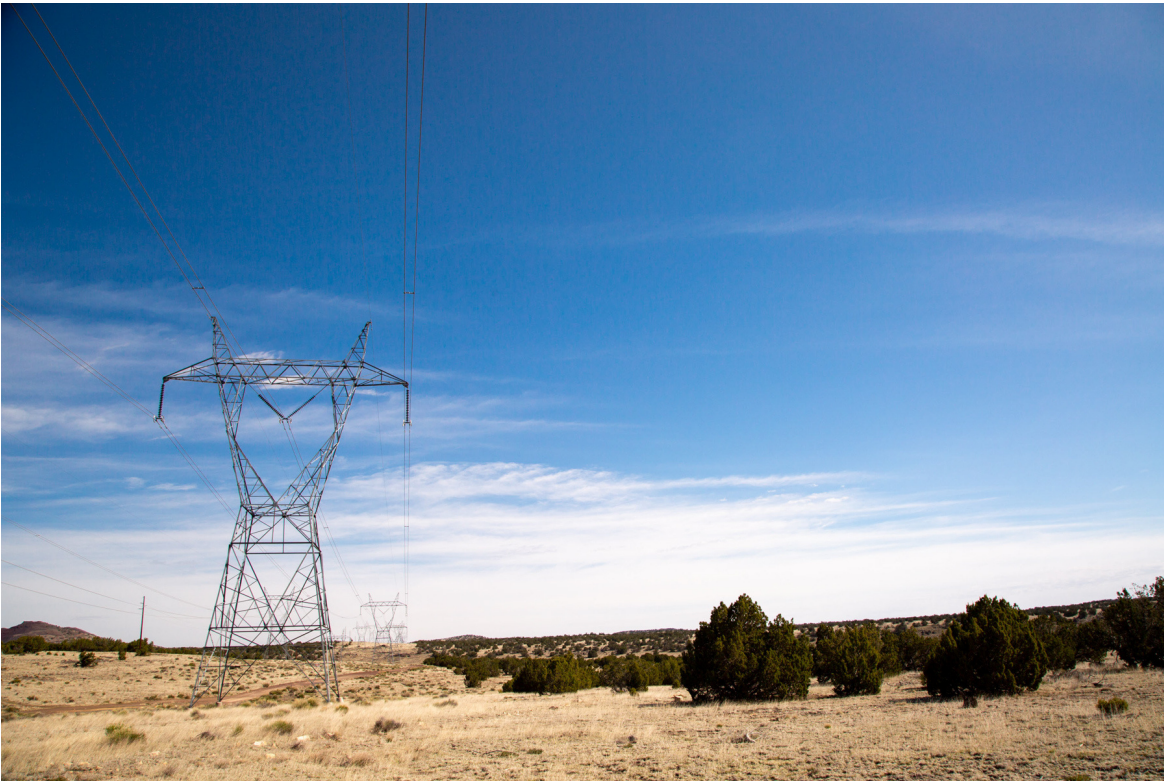
345 kilovolt line outside of Flagstaff, AZ in WAPA's Desert Southwest Region. Credit: U.S. Department of Energy – Western Area Power Administration, File Photo
